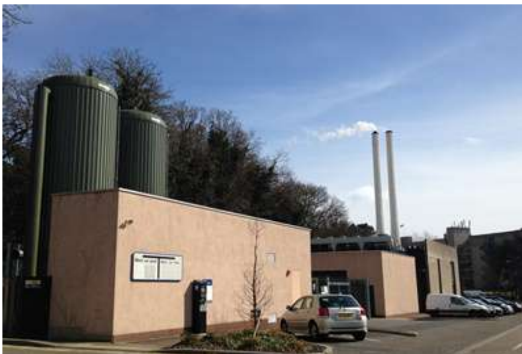
Figure 5 Thermal Storage System at UEA
