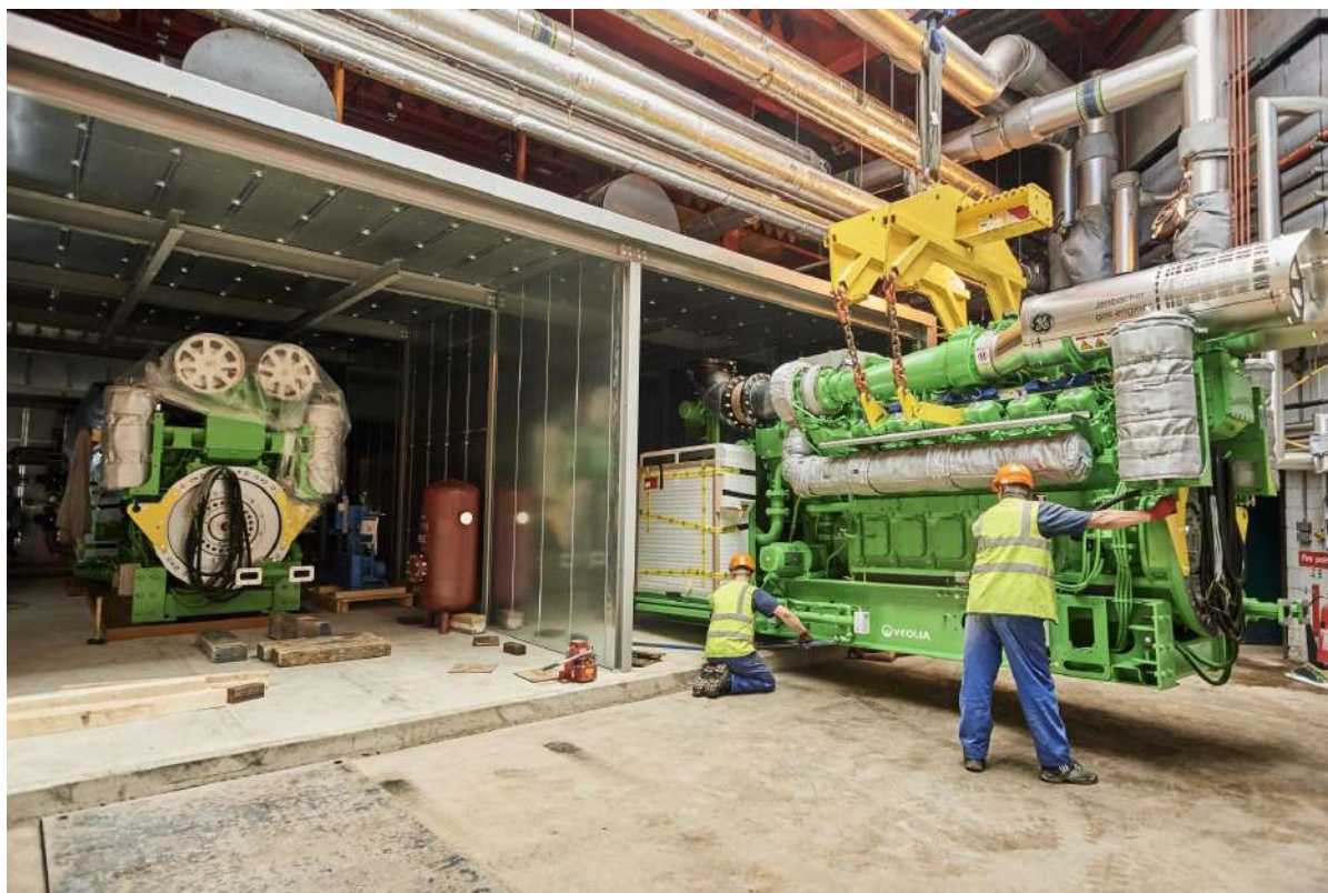
Figure 3 New CHP units installed at UEA
