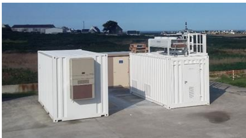
Figure 2 : Photograph of the Ouessant electricity storage facility
